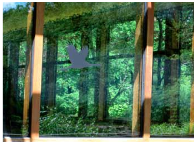
A single decal is ineffective for collision prevention on a window of this size, as birds will simply attempt to fly around it. Photo: Christine Sheppard, ABC
